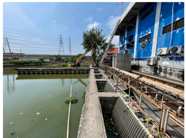
Fig. 7. water retention and pumping station (2022).
