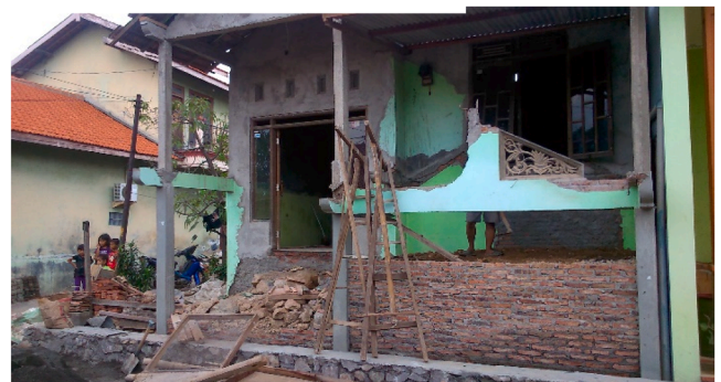
Fig. 6. Ground floor is given up, residents demolished and rebuilt their house to be able to cope with tidal floods (2013).
